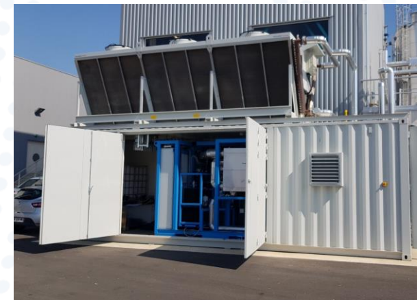
Heat recovery on Incinerator– 180kW ORC - France
