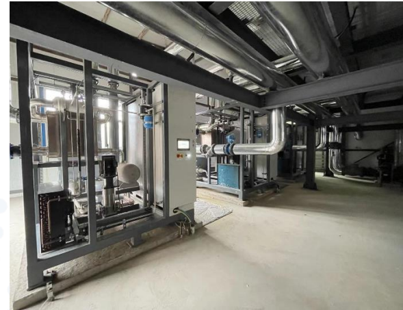
Heat recovery on Geothermal well – 3 x 100kW ORC - China
